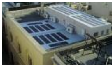
Fig. 3. The membrane incorporating PV elements as installed on the roof of Palazzo Falson
